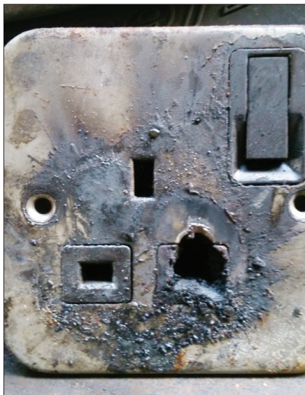
Water blown in through a leaking skylight and onto the charger's lead shorted the plug
