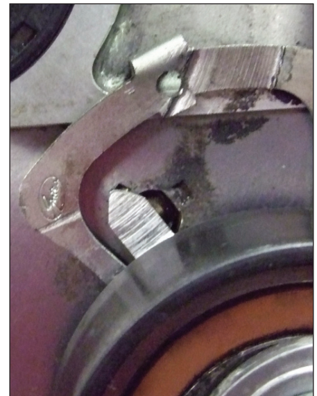
The upside down tensioner left no clearance room for the timing belt, as can be seen by the scoring in this picture
