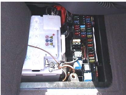
Picture 1 Fuse box
