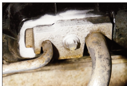
Frost on the expansion valve or vents can be caused by an expansion valve failure
