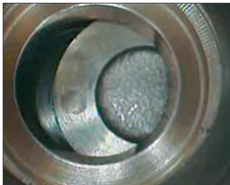
Valves can be examined by inserting the probe in the spark/glow plug hole
