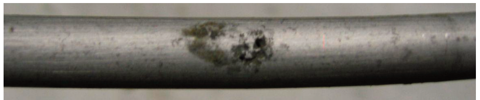
A pin-hole leak on a fuel line was sucking air into the line, but wasn't leaking diesel yet
